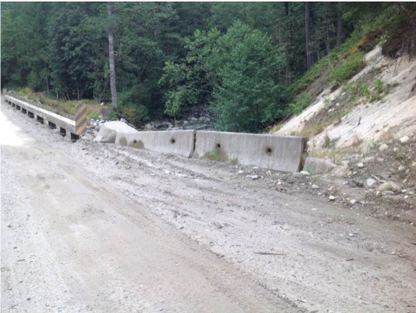
left bank concrete no posts pointing wrong way
