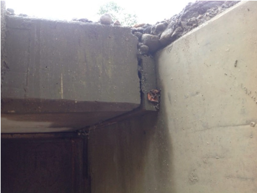
gap between right ballast wall and deck filled with treated 2x6
