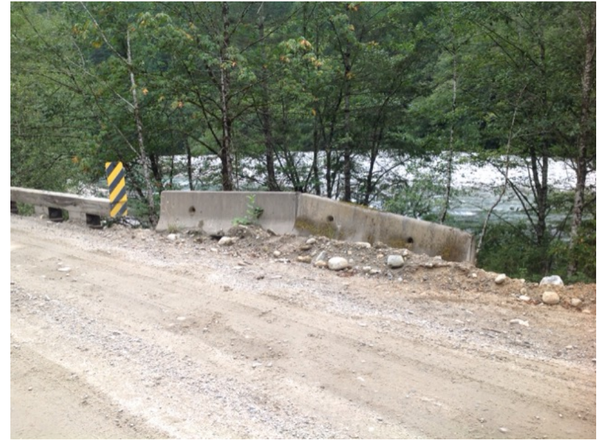
right bank downstream no post barriers
